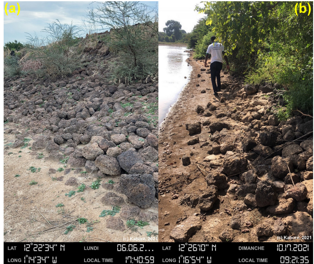
Figure 5. (a) Disorders on upstream riprap, Koala dam (Centre Region). (b) Disorder on upstream riprap, Siga dam (Centre Region).
