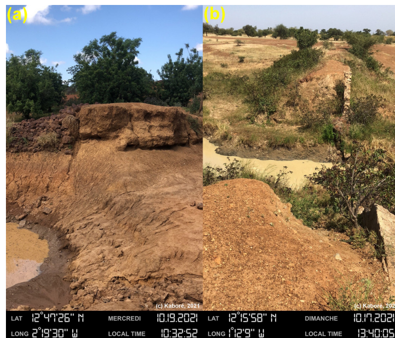
Figure 10. (a) Transverse cracking, Salouf Boulssi dam (Centre Region). (b) Transverse cracking, Veh dam (Northern Region).
