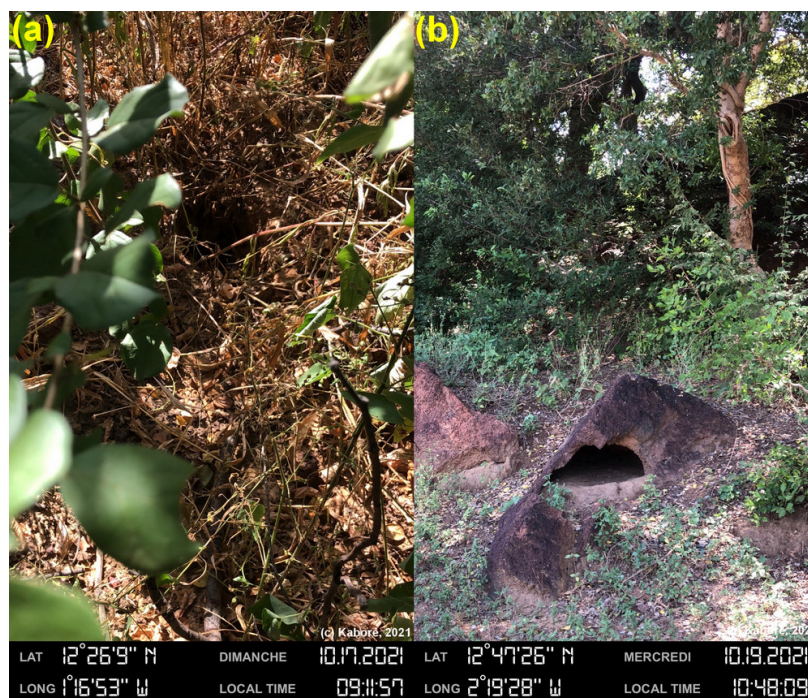
Figure 7. (a) Presence of burrows on the dam due to rodents, Siga dam (Centre Region). (b) Presence of burrows due to digging crocodiles, Veh dam (Northern Region).
