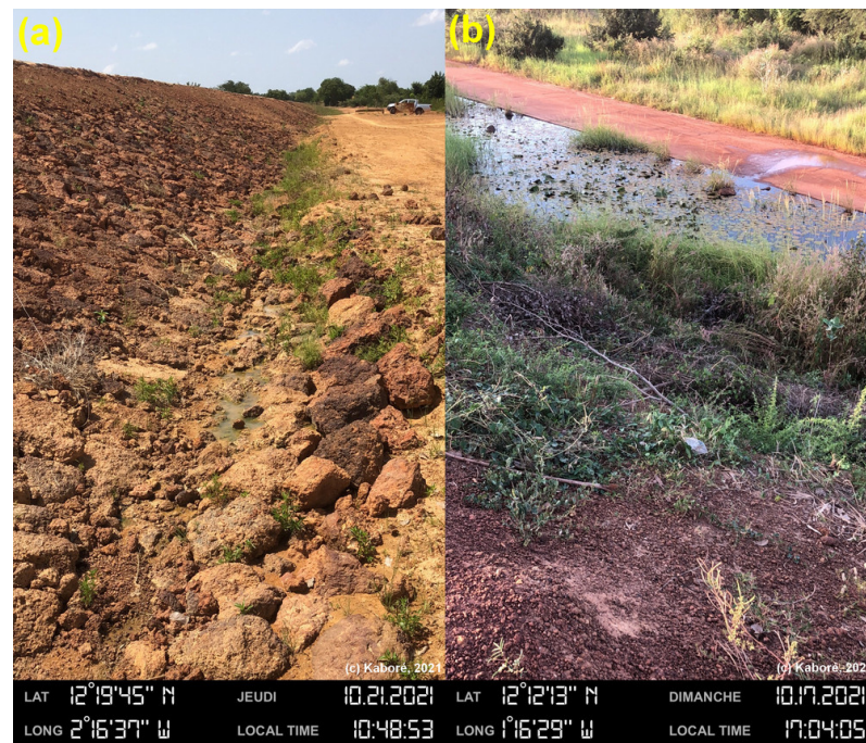
Figure 9. (a) Presence of slight leak in the upstream-downstream direction, Doulou dam (Centre-West Region). (b) Presence of slight leak in the upstream-downstream direction, Ramogwende dam (Centre region).
