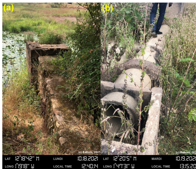
Figure 12. (a) Aging intake structure, Petit Tansobentenga dam (Centre Region). (b) Aging intake structure, Taama dam (Centre Region).
