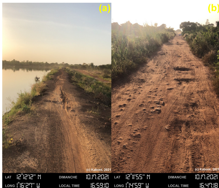
Figure 6. (a) Anthropogenic erosion of the platform, Ramogwende dam (Centre Region). (b) Anthropogenic erosion of the platform (due to vehicle passage), Ridrin dam (Centre Region).
