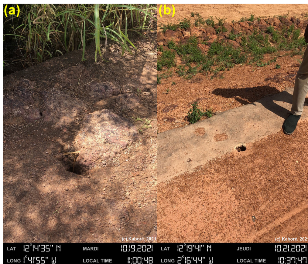
Figure 13. (a) Orifice on crest causing internal erosion, Doulou dam (Centre-West Region). (b) Orifice on crest spillway causing internal erosion, Koakin dam (Centre Region).
