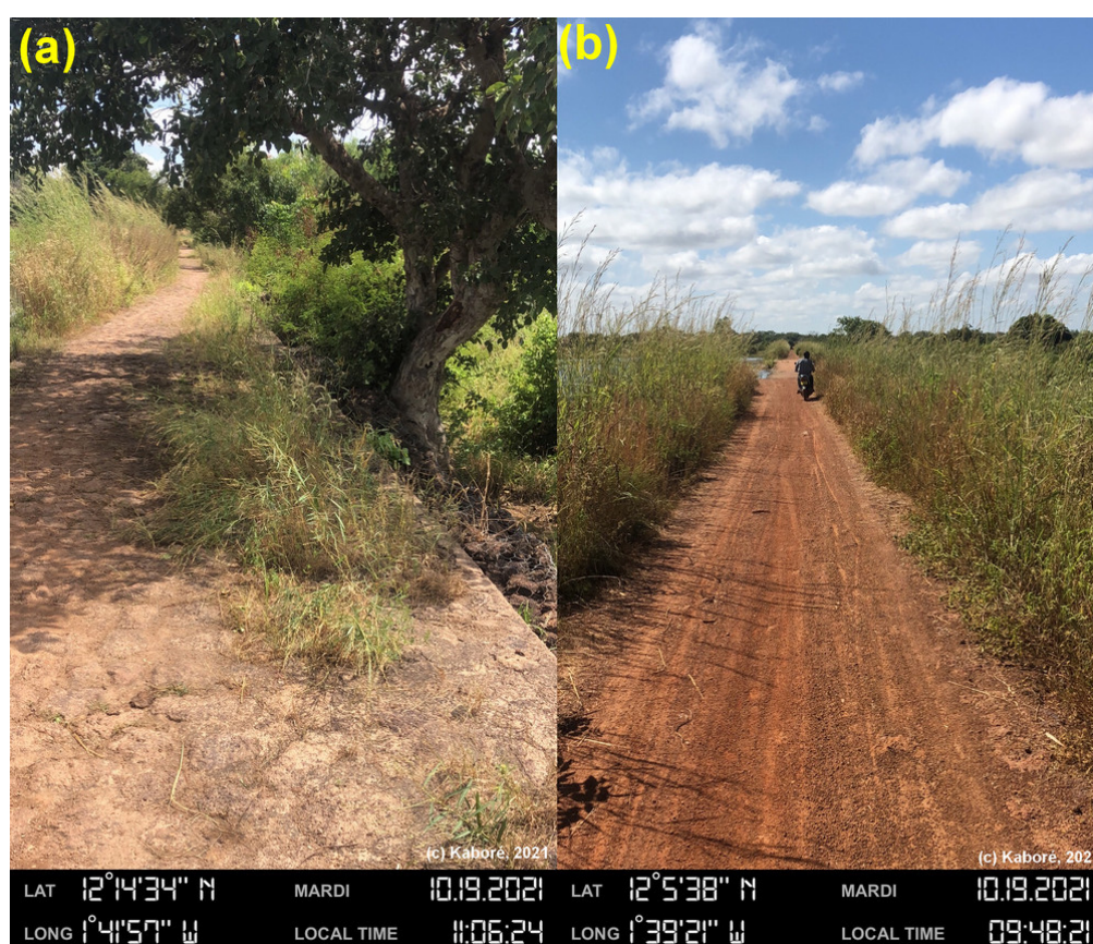
Figure 8. (a) Vegetation on dam and spillway, Koakin dam (Centre Region). (b) Vegetation on upstream and downstream slopes, Kalzi dam (Centre Region).
